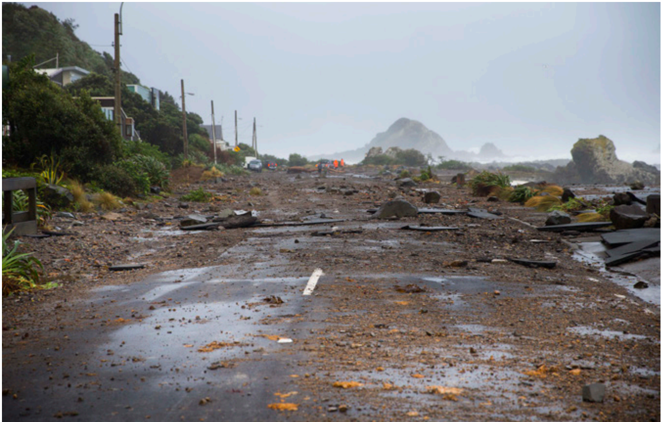
In 2013, a severe southerly storm caused widespread damage along the south coast of New Zealand's North Island
