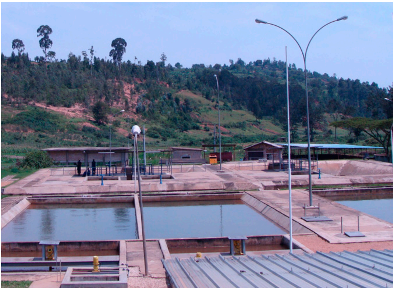
Butare city water supply, Republic of Rwanda. This project aimed at providing Butare city with its potable water needs and improving the local population's health by reducing the risk of waterborne diseases
