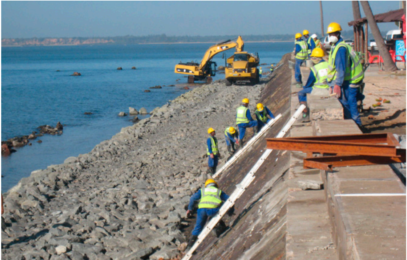
Maputo City coastal protection, Republic of Mozambique. The project falls within the government programme for the development of infrastructure in the capital, Maputo, and the project aims at the prevention of the continuous erosion of Maputo coast, for the protection of public and private properties and prevention of deterioration of the environment
