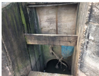
Part of colonial sewer network in Kratie's city center
