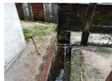
Insufficient sewer system
